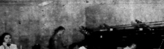
IRONING OUT YOUR TROUBLES—In any new installation as large as the Morehead dial system there are bound to be gimmicks. Some phones were out and others didn't dial properly Sunday morning. But, these are rapidly being worked out by the crew and others. General has some of its key personnel in Morehead this week to handle these initial problems.
