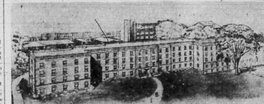
NEW HOME FOR UK GIRLS—Construction is under way on this modern residence hall for girls at the University of Kentucky, and it is expected to be ready for occupancy in the fall. The $1,250,000 building is being financed through a $200,000 gift from the Keesel Foundation, a $720,000 loan from the federal government, and the remainder from accumulated earnings in the UK plant fund. More than 300 women students will be housed in the four-story structure.
