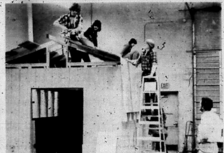
Burt Blankenbecker, right, the instructor in the carpentry class at the Rowan County Area Vocational Education Center, supervises the construction of a Dutch Mini Barn, which can be used as a utility building and/or work shop. Students on the roof are left to right, John Leone, 17, Doug Easton, 17 and David Manning, 16. (Staff photos by Mark Perkins)
