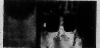
This electrical unit at the Morehead State University switchgear station on University Street exploded and caught fire Sunday morning, blacking out most of the campus. Electrical service was expected to be restored by late today. (Morehead State University Photo)
