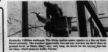
Kentucky Utilities workman Tim Hicks makes some repairs to a line on Main Street recently. The weather apparently was not any warmer up there than on ground level, as Hicks didn't stay very long. So much for the saying that hot air rises. (Staff photo by Kathy Partin)
