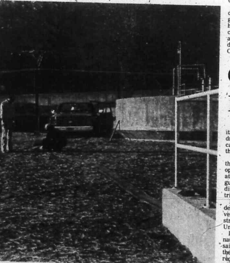
Sonny Barker, Norm Bowling and Gary Thompson, of Shook Contractors, worked this week to decommission the old waste water treatment plant in Morehead. All the flow into the old plant has been diverted into a new facility at Bluestone. Waste from the old tanks is being pumped here into a new collector in the foreground. (Staff photo by Joe Lamb)
