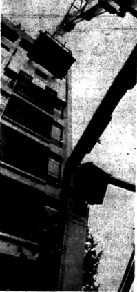
Workmen recently bolted a ground plane antenna on Anderson Hall at the 6th floor.
