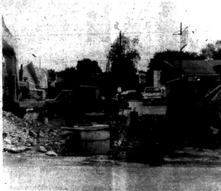
IF YOU'VE BEEN WONDERING why there is a hole in the road on Math Street in Mt. Sterling, let us explain. The excavation is part of the new sewer expansion project currently being undertaken by the city. (Staff Photo)
