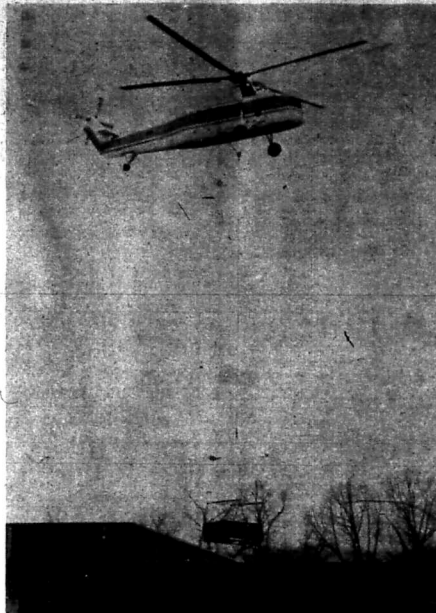
DOING IT THE EASY WAY . . . This crew from the Carson Helicopter Company spent much of Monday morning lifting air-conditioning units onto the roofs at Morehead's Trademore Shopping Center. The pilot said the crew of three had just completed a similar job in Tennessee over the weekend and has worked in just about every state east of the Mississippi River. The first retail store to open in the center will be Malone's which plans to open at noon Sunday, March 19. Trademore's first business, the Windmill Restaurant, opened several weeks ago.
