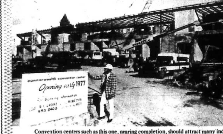
Convention centers such as this one, nearing completion, should attract many industries to Kentucky.
