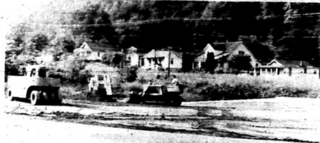
NEW BRIDGE . . . A move is accelerating for a modern highway connecting the Mountain Parkway and I-64 at Morehead. As a first, although minor, step this bridge on Morgan Park near the Oscar Caudill home and service station, is being re-built to wider standards with new approaches. Workmen started this week on the project. The new highway would follow, to an extent, the path of the Morehead and North Fork railroad from Paragon in Rowan County.
