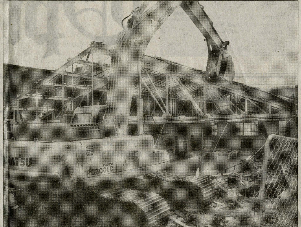
Vanessa Overholser photo Morehead State University's historical pool building is in the process of being torn down. The building was established in 1933 and it was used until 1988. The Solid Rock Construction Company, West Portsmouth, Ohio is working on the demolition of the old building. This disassembly began Dec. 27 and the process is expected to be completed within two weeks.
