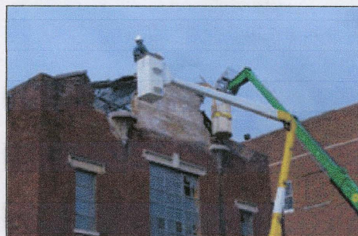
Workers carefully removed the 30 pieces of sculpted limestone which formed the distinctive frieze on the facade of MSU's Senff Natatorium.
