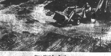
10,000 seat stadium, an eight-lane all-weather track, a baseball field and practice football field. Construction is expected to be complete in late August.
