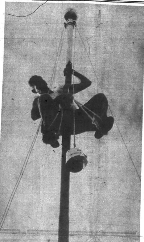
So You Think Your Job's Hard? Harold Williams of Boone, N.C., looked comfortable as he painted the flag pole at the Morehead Post Office Tuesday, it's a safe bet that not everybody would change places with him. Williams is employed by Gallimore Construction Co., of Greensboro, N.C., which is doing a renovation job on the Post Office here.
