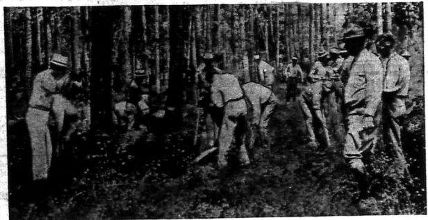
President Roosevelt at Hyde Park pushed a button that started preliminary work on the Florida ship canal that will connect the Atlantic with the Gulf of Mexico. In this picture are seen men under army supervision cutting down trees to clear the way for the big channel.
